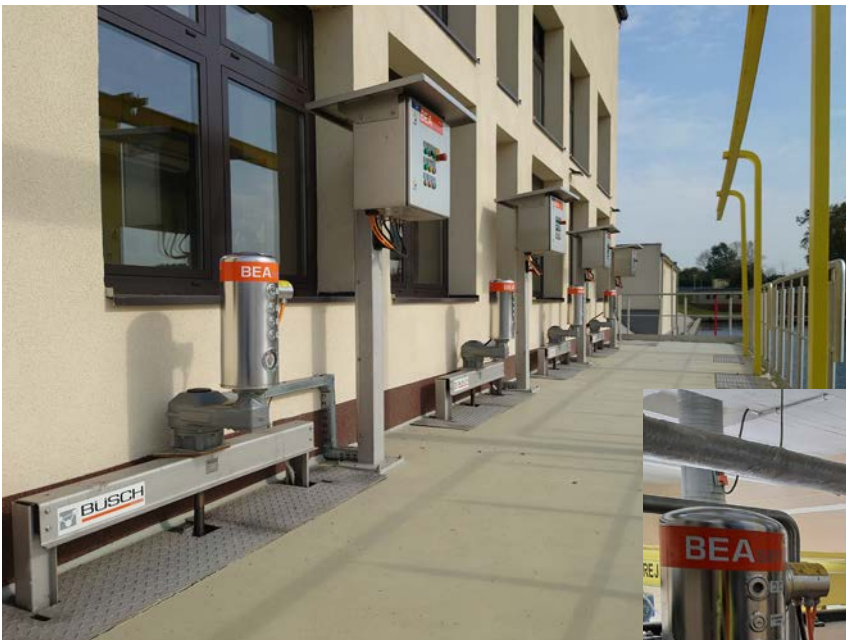
PUMPSTATION ZERO – WARSCHAU, POLEN PUMP STATION „ZERO” – WARSAW, POLAND
