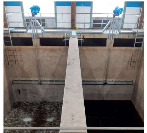
Double rotary weir with front control with electric drive. Wastewater treatment plant, Germany
